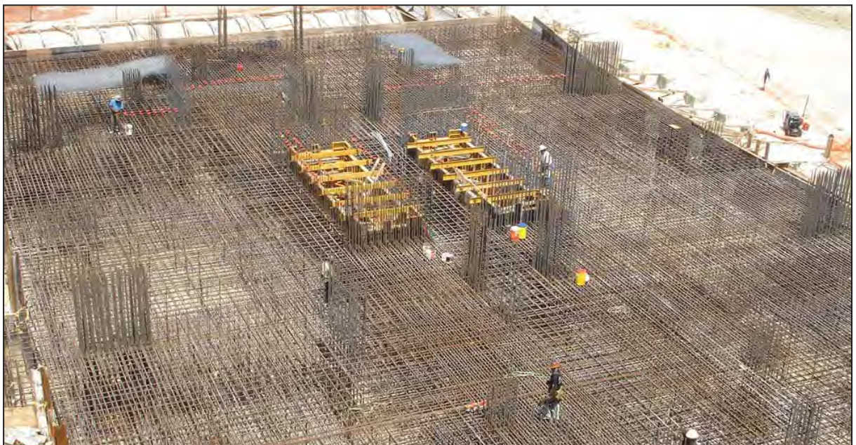
Mat foundation reinforced with MMFX 2 bars for a 50-story high-rise in Miami, FL.
